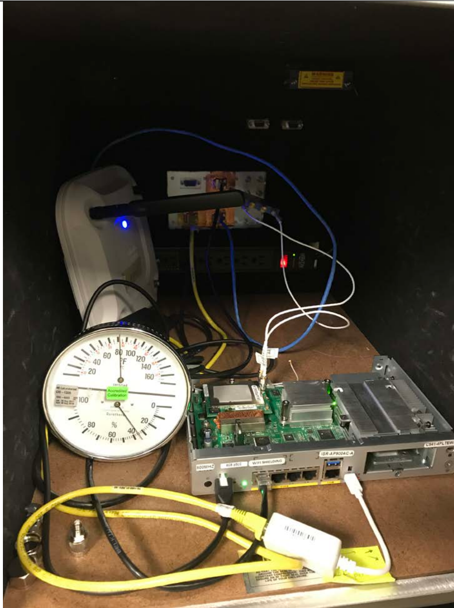
Title: DFS Setup: C1101-4P-LTEP-Wx connected to test system, along with companion device and environmental monitor, inside shield enclosure.
